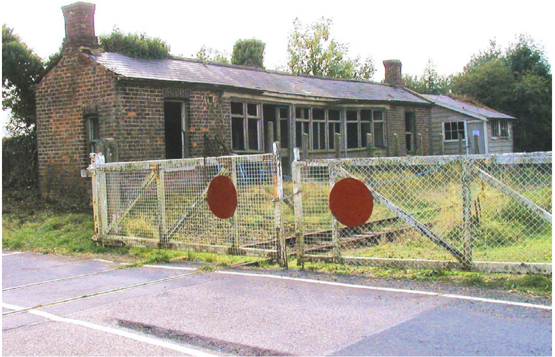
ABOVE: The current condition of Scruton station buildings, having been in touched for many years. Scruton Parish Council
